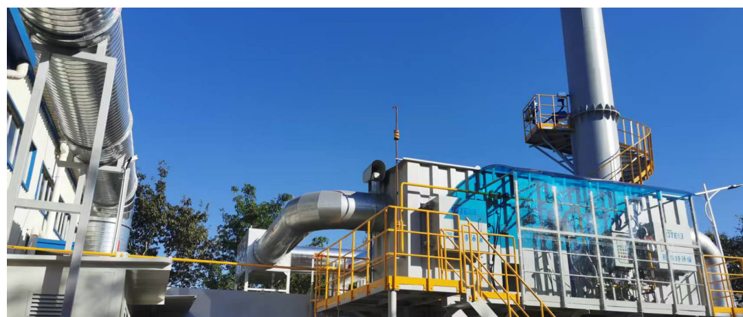
1 VOCs treatment facility
