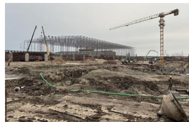
Part of the plant before the retrofit
