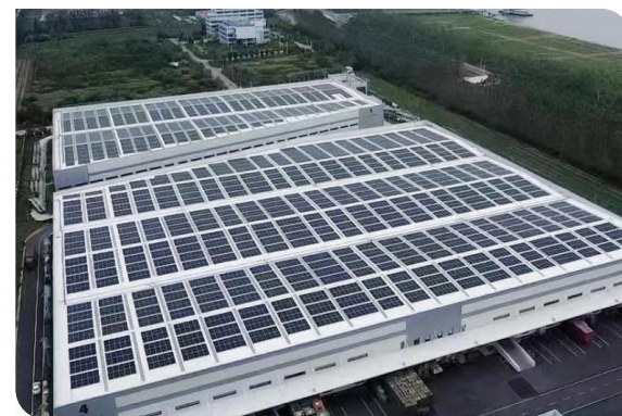
Hannan Jieyuexing Photovoltaic Power Project
