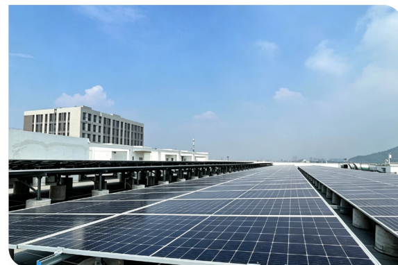
Photovoltaic panels at Keerun Warehouse
